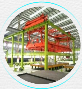
Installation and Commissioning 设备安装服务
